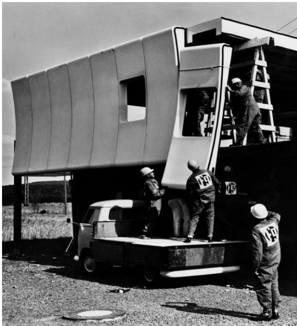
Fig.4 shows the FG (fiber glass) 2000 project in Germany; the individual elements are sandwich elements with 4-6 mm thick GRP layers either side of a 60 mm thick rigid Polyurethane foam core [10].
