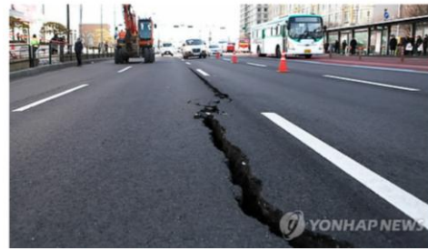
(b) First road crack
