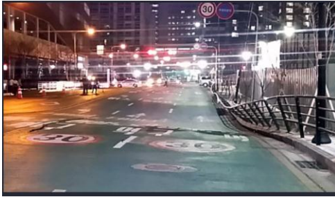
(c) Second road crack and settlement
