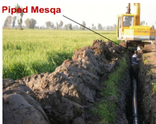
Fig. 3. Improved Pipeline Mesqa
