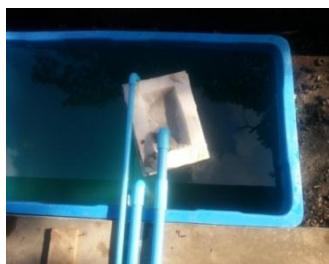
Fig 5 Water Recycle Tank
