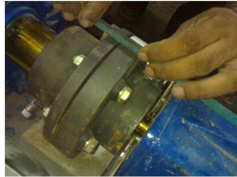
Fig. 8- Alignment of pump and motor
