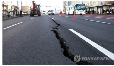
(b) First road crack
