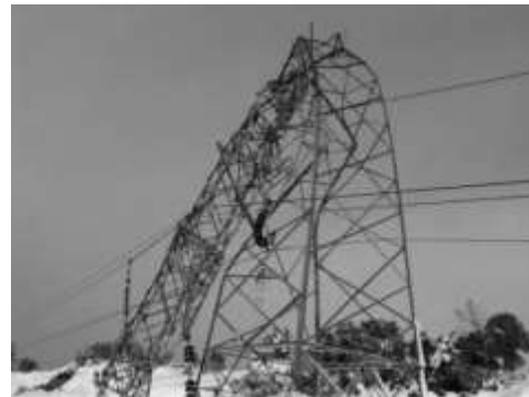
Fig. 2 The damaged ETL pole
