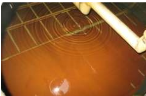
Fig.6. Bed's Condition of Anion Exchanger
