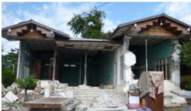
Fig. 3 Collapse of masonry walls in single-storey governmental office
