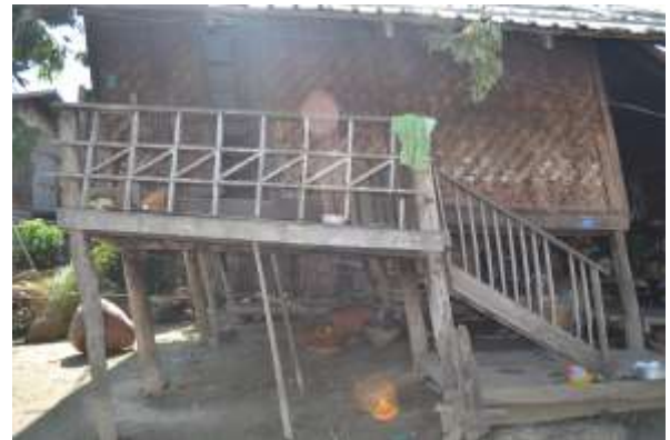
Fig. 5 Failure of veranda in wooden residential building
