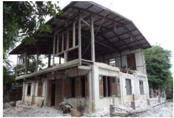
Fig.4 Collapse of masonry walls in two-storied residential building
