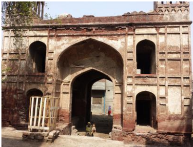
Fig. 7 Scaling seen inside the ghalibkari
