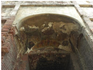
Fig. 1 View of the pishtaq entrance showing cracks
