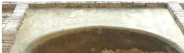
Fig. 14 Cracks in the super structure
