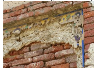
Fig. 5 Scaling seen inside the ghalibkari
