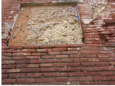
Fig. 12 Defects due to acid rain on the exterior
