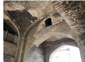
Fig. 3 Scaling seen inside the ghalibkari
