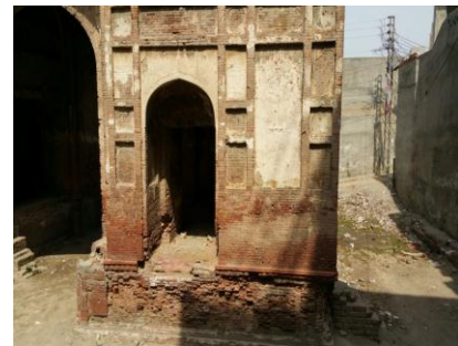
Fig. 10 Massive contour scaling noticed on the front facade
