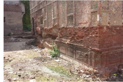
Fig. 16 Damage done in the surrounding of the structure
