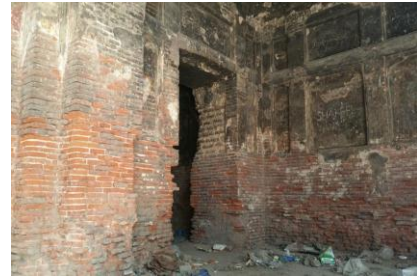
Fig. 15 Damage done in the inner chambers
