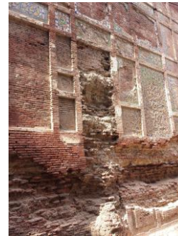
Fig. 4 Contour scaling seen on the façade
