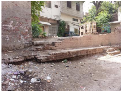
Fig. 8 Massive contour scaling noticed on the front facade
