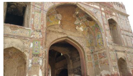
Fig. 6 Massive contour scaling noticed on the front façade
