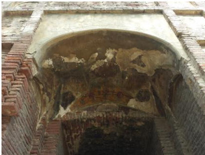
Fig. 13 Defects due to acid rain on the fresco work
